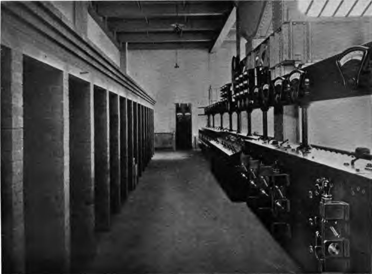
OPERATING GALLERY IN SUB-STATION
